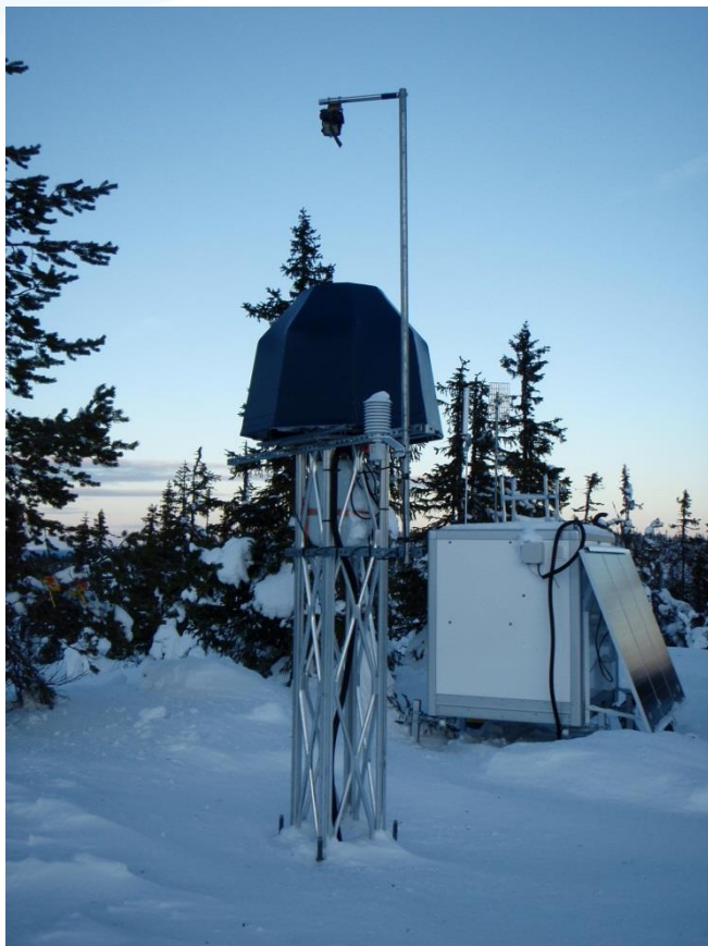
Installation in Cold climate (October in Northern Europe)
